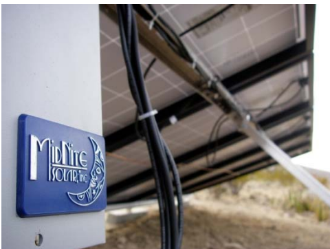
Left: Combiner installed on A pole mount array.
