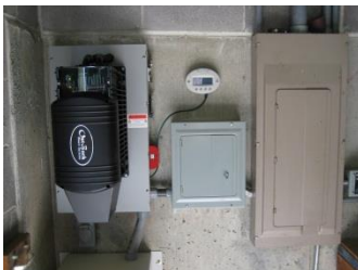
A Jay Peltz installation, CA In the basement
